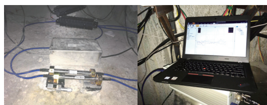
(c) 在线校准系统安装现场 (c) In-situ installation of online calibration system
